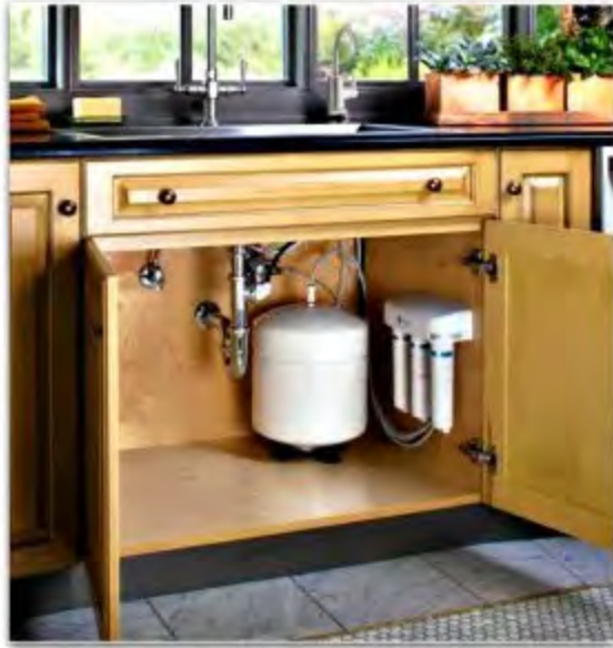
Figure 15. Example of POU RO treatment.
